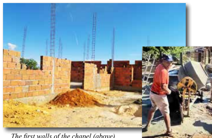
The first walls of the chapel (above) and Fr. Adilson mixing cement (right.)
